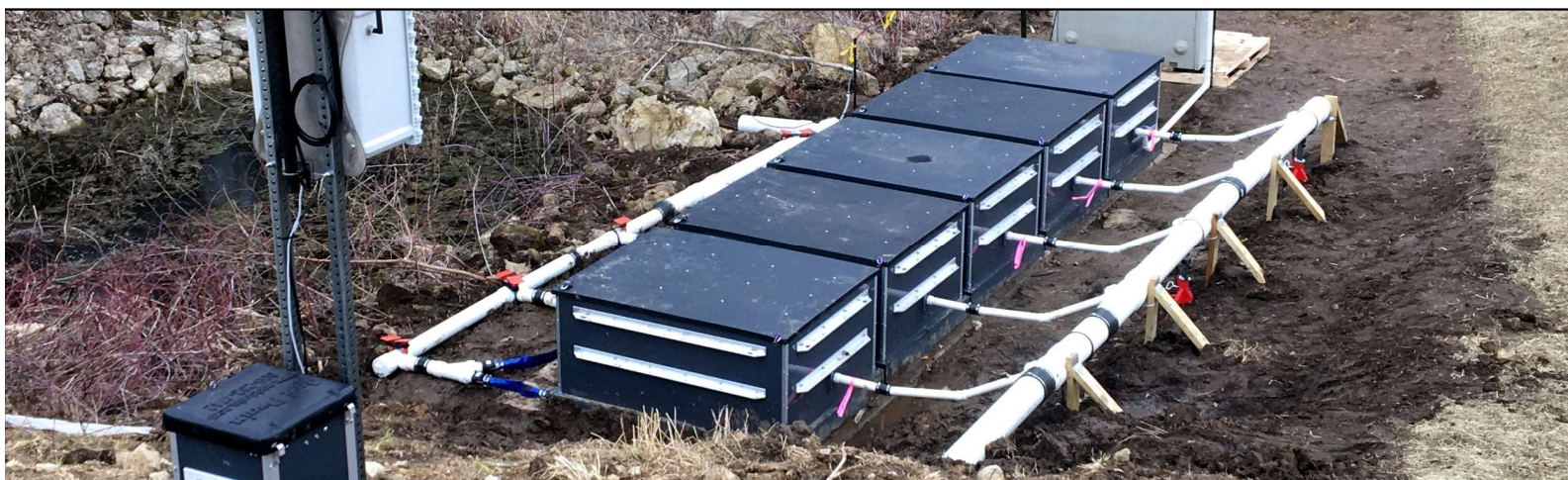
Figure 2. CAPTure™ installation with boxes in parallel for runoff and tile treatment of 100 acres. (See: https://youtu.be/POPVedDvZg8?si=E04diP9Qpyie5a3e&t=127 )
