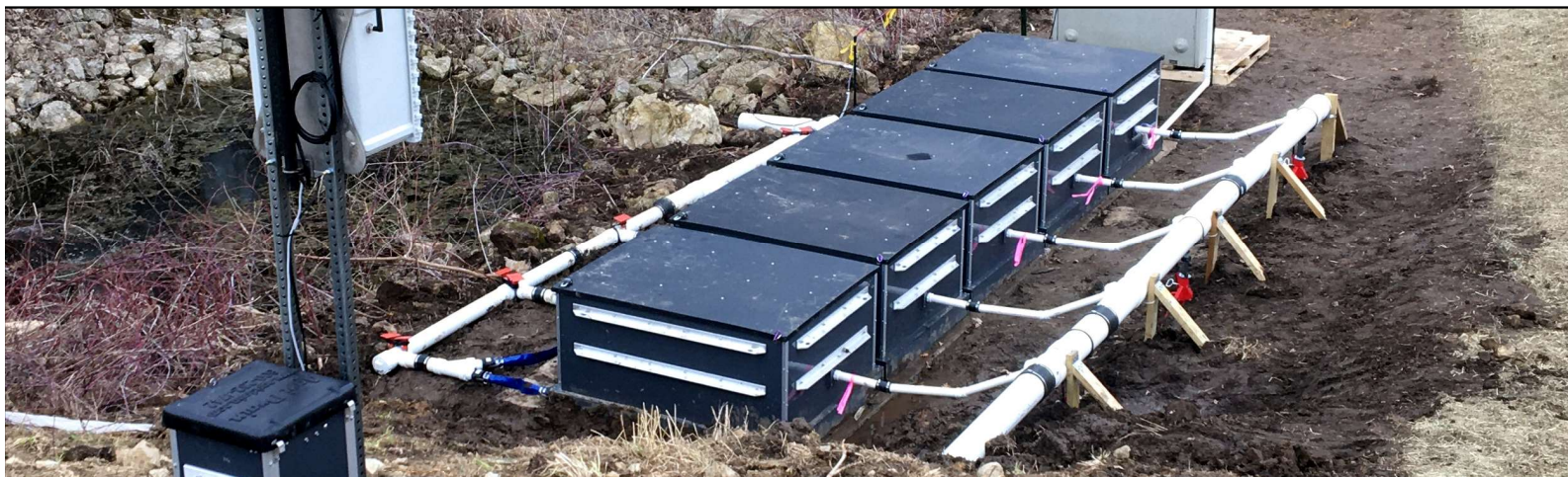
Figure 4. CAPTure™ installation with boxes in parallel for runoff and tile treatment of 100 acres. (See: https://youtu.be/POPVedDvZg8?si=E04diP9Qpyie5a3e&t=127. )
